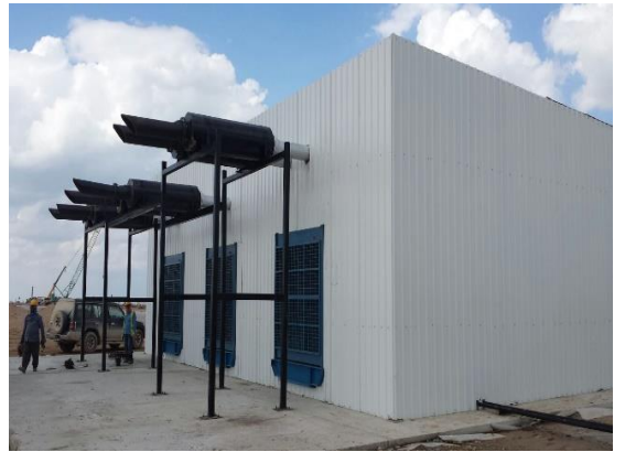
Power Generator House
