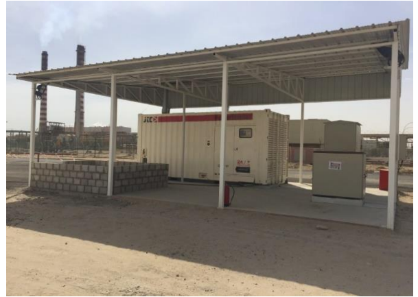
Generator Shelter - DOOSAN
